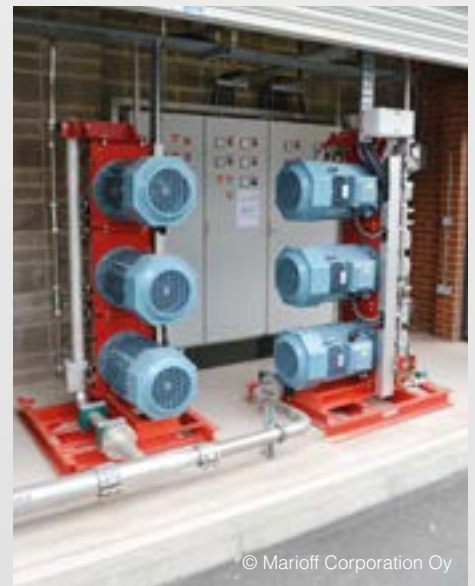
The modular pump units and control panels to the rear.
