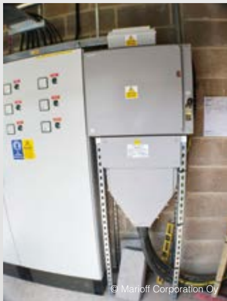
Control panels and dedicated incoming electrical supply.
